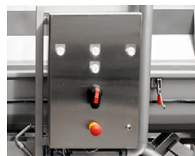
Standard screw conveyor electrical/operator panel.
