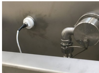
Valve shown mounted on mixer. Temperature sensor shown to the left and valve shown to the right.
